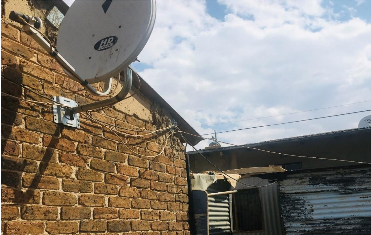
Figure 29: Electrical Connections to backyard rooms (Photo by Chabalala, 2019)
