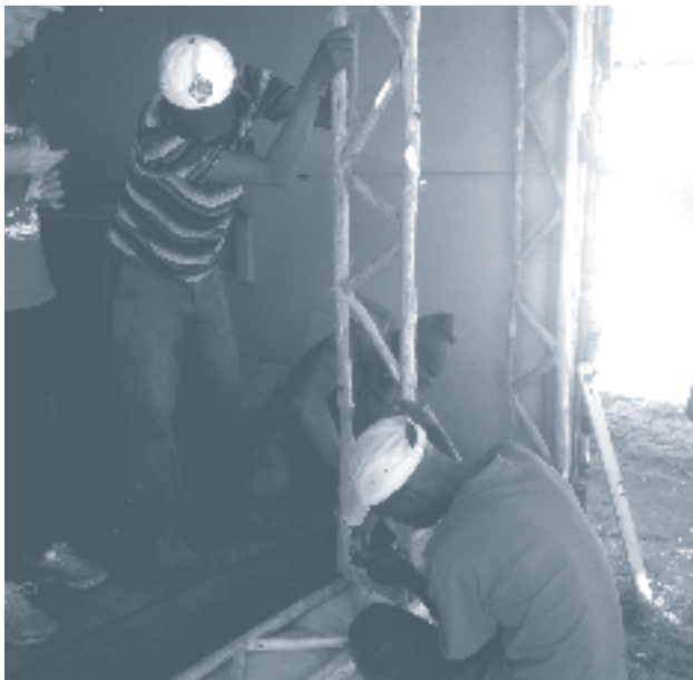
Setting up of a frame on the foundation – training day Zweledinga 17 September 2013
